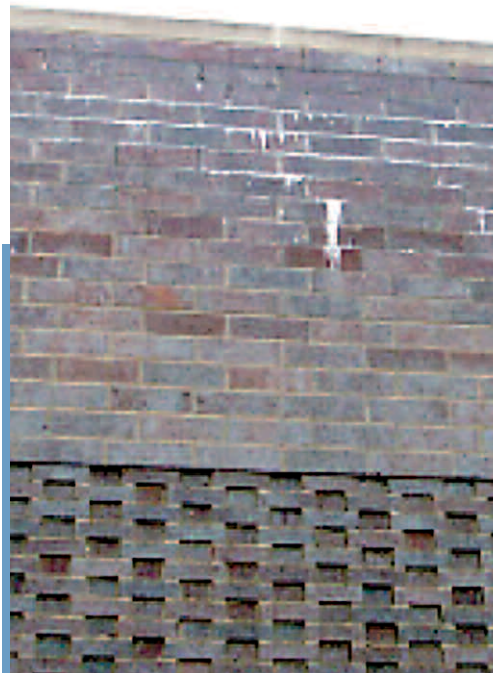
Note the efflorescence, and the flush limestone cap- it should have had 1 1/2” projection, with drip edge and flashing under the cap.
