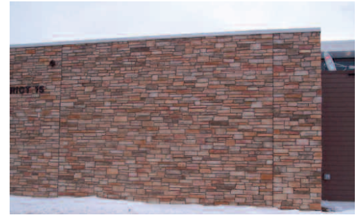
Picture 2. Adhered veneer with movement joints properly installed. By code, these movement joints must be shown on the drawings.
